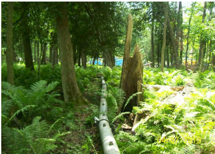
Temporary water pipe strung through wooded area (River Road East dead end)
