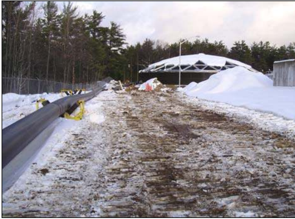
The 500-mm diameter watermain stung through the Water Pollution Control Plant, ready to be pulled under the Wasaga Beach Provincial Park property.
