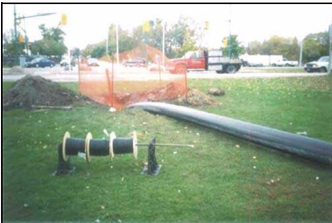
Hydrant lead beneath Lakeshore Drive.
