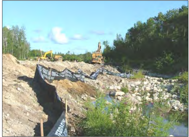
The existing creek bed (at the right) was protected while construction of the new alignment continued.
