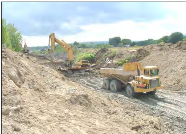
Heavy equipment beginning the excavations for the channelization of the creek in the spring of 2004.
