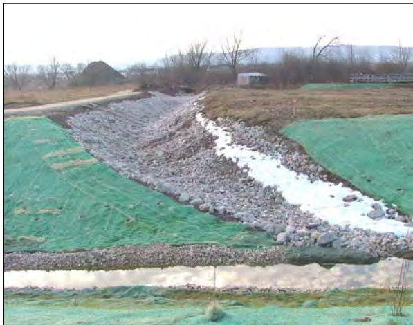
A weir was constructed at the original merging point of the Petun to divert flow into the new stream bed.
