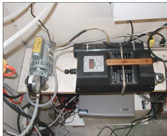
Figure 5 – Rotronic Temperature/Humidity Transmitter (incoming sewer air)
