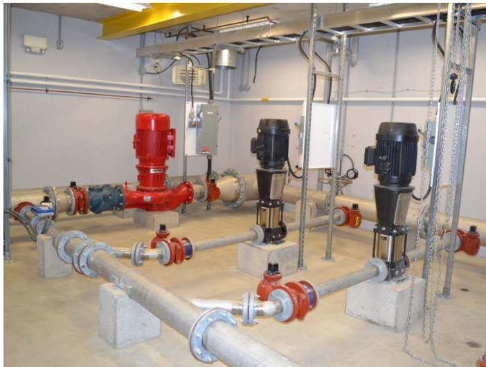
New Water Booster Station pumps.
