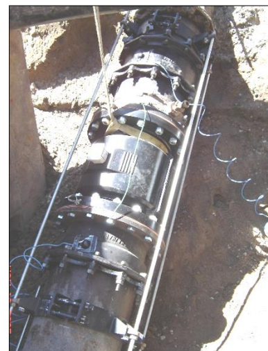
Electromagnetic flow meter positioned on the common fill/draw line
