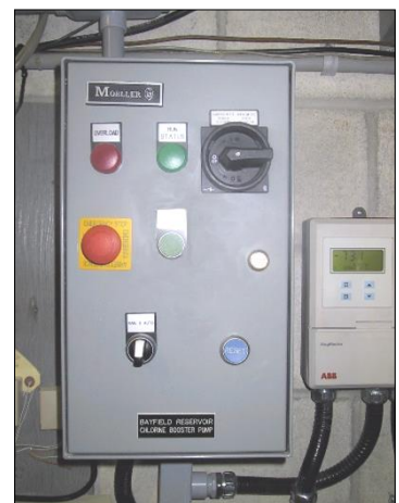
Bayfield Street booster-pump control and monitoring equipment.
