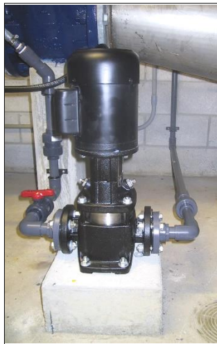
The chlorine booster pump at the Bayfield reservoir showing the water draw and injector piping.
