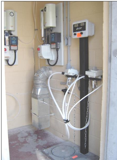
Inside the chlorine room at the Anne Street reservoir showing the chlorinators, weigh scales, vent and gas sensors.
