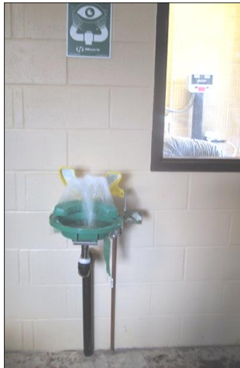
The emergency eye-wash station on the outside wall of the chlorine room.
