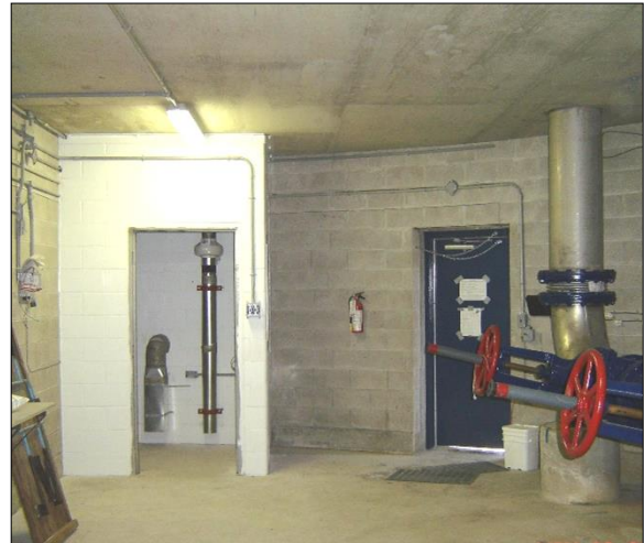
Completed chlorine room inside the valve room at the Mapleview Elevated Tank Reservoir.
