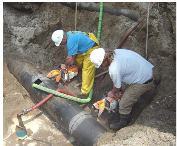
Construction personnel cutting a section of the common fill/draw line to provide a space for the flow meter at the Mapleview Elevated Tank.
