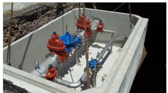
Use of a prefabricated pressure reducing valve (PRV) chamber reduced installation time and minimized disruptions.
