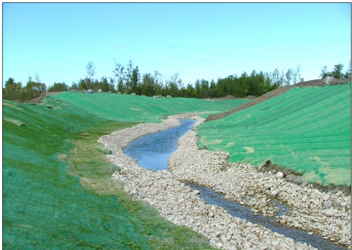
A completed section of Phase III of the Black Ash Creek Flood Control Project showing the seed and erosion control blankets on the side slopes.
