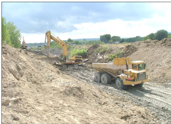
Heavy equipment beginning the excavations for the channelization of the creek in the spring of 2004.
