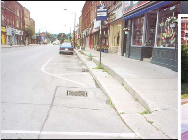
The existing road surface and sidewalks of Sykes Street in Meaford were showing signs of deterioration in 2004.
