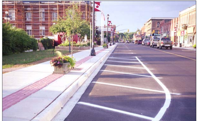
In July of 2005, the watermains have been replaced and the new road surface is finished. New sidewalks with colour patterned concrete, new curbs and gutters, street lighting and streetscaping completed the road restoration.
