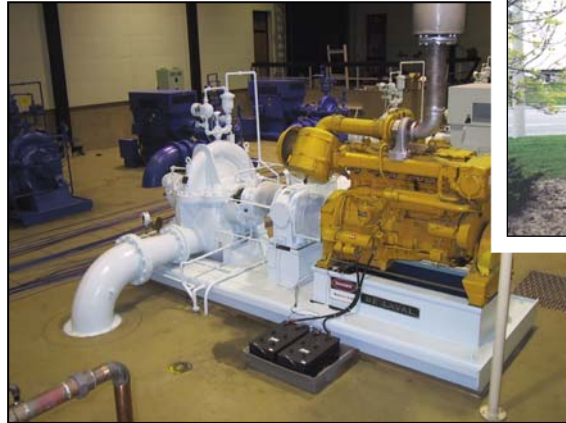
Pump No. 4 at Herridge Pumping Station
