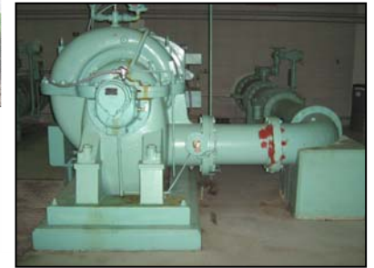
Pump No. 6 at Hanlan Pumping Station (above)
