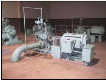
Pump No. 6 at East Brampton Pumping Station (above)
