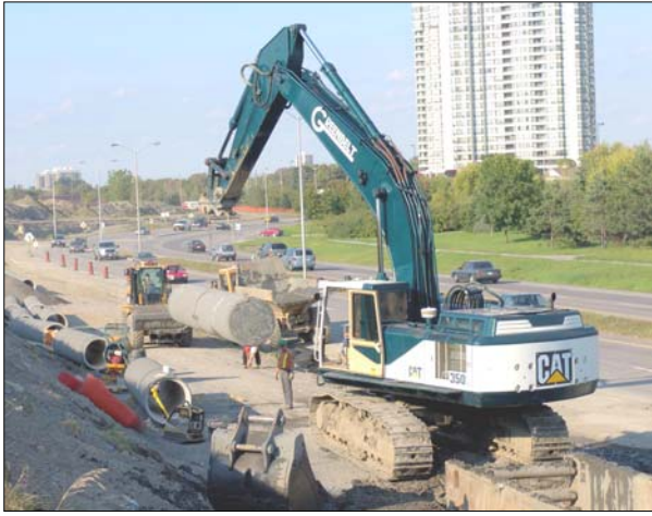
The majority of the 3.9 kms of watermain was installed using traditional trenching methods.
