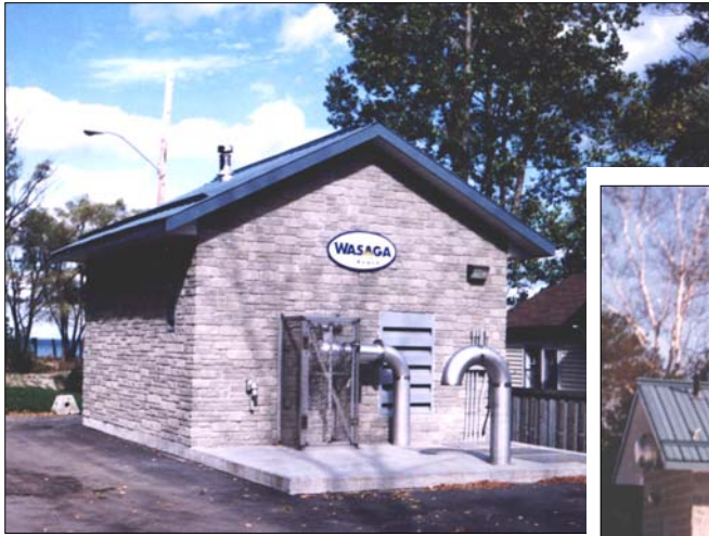
Pump Station No. 1
