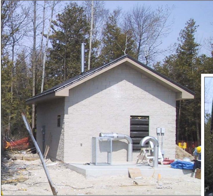
Pump Station No. 15 under construction in the west end of Wasaga Beach.
