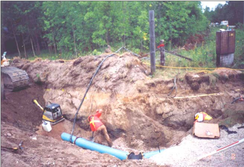
Laying the 300-mm diameter forcemain – a component of Phase 1 of the multi-stage expansion.
