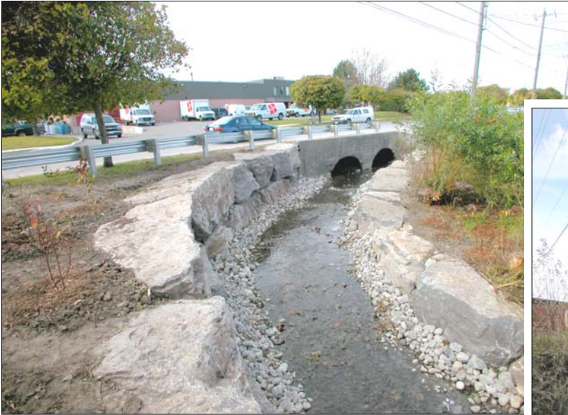
Completed stream-bank restoration at Enford Road showing armour stone placement and the channel lined with river-run stone lined.
