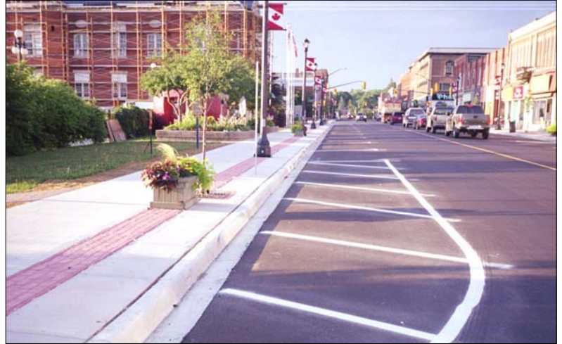
In July of 2005, the new road surface is finished. New sidewalks with colour patterned concrete, new curbs and gutters, street lighting and streetscaping completed the road restoration.
