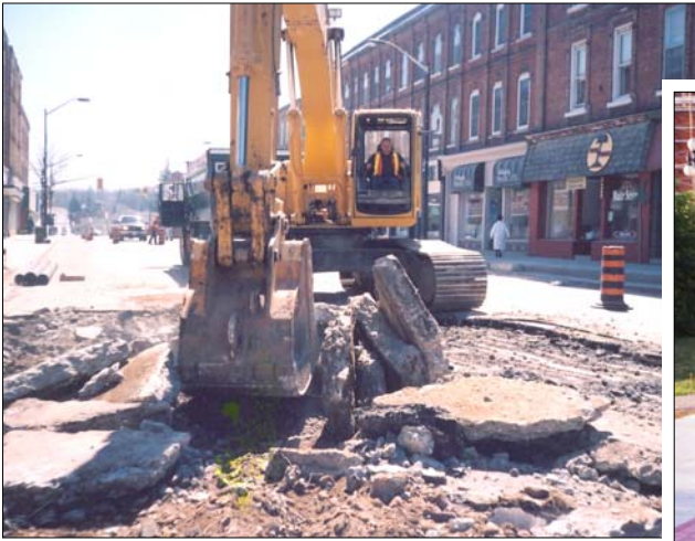
During the early part of construction, a 20-mm layer of reinforced concrete was discovered under the existing asphalt.
