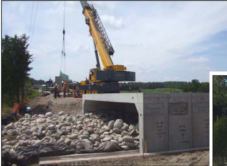
Photos showing the installation of precast concrete bridge units and the completed bridge and roadworks.
