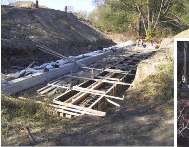
These photos show the new footings at the base of the excavation, the first two precast concrete units being lowered into position and the bridge structure with five sections in place.
