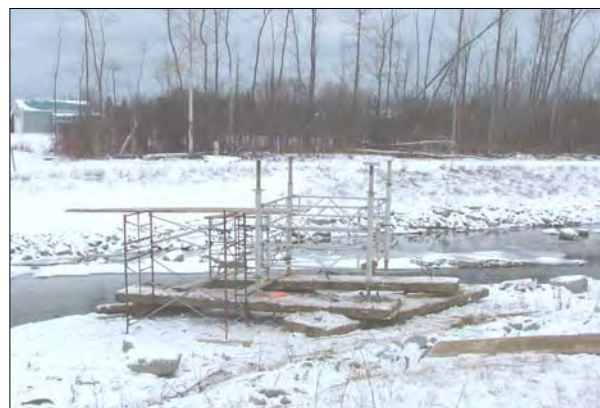
A temporary scaffold and support structure was erected on the floodway channel bed.
