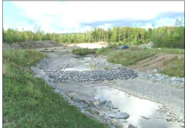
A silt cofferdam was constructed at the upstream limit of Phase II to prevent sediment migration.
