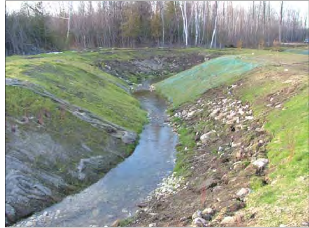
A completed section of the new Petun branch meandering stream bed, which parallels the main channel for 500 metres
