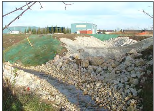
This photo shows one of the rock revetments, completed slopes and landscaping.
