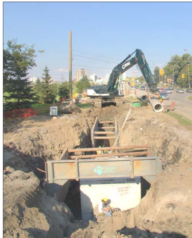
The majority of the 3.9 kms of water main is being installed using traditional trenching methods.
