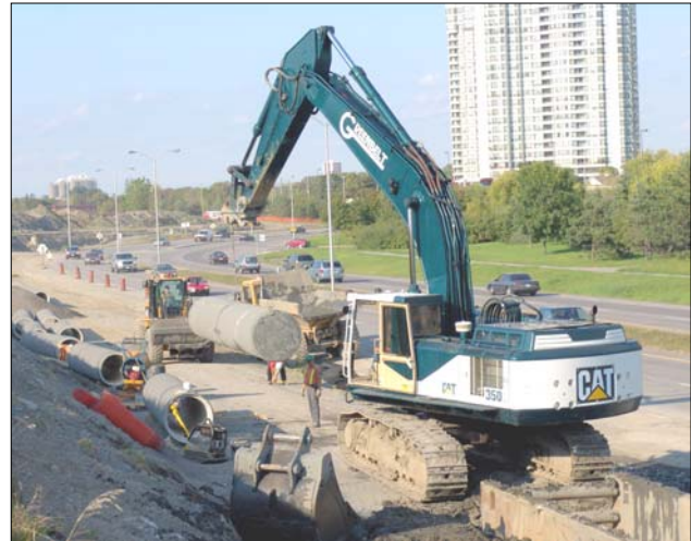
By installing the new trunk water main off the traveled portions of the four-lane divided roadway (Riverside Drive), traffic disruption was kept to a minimum.
