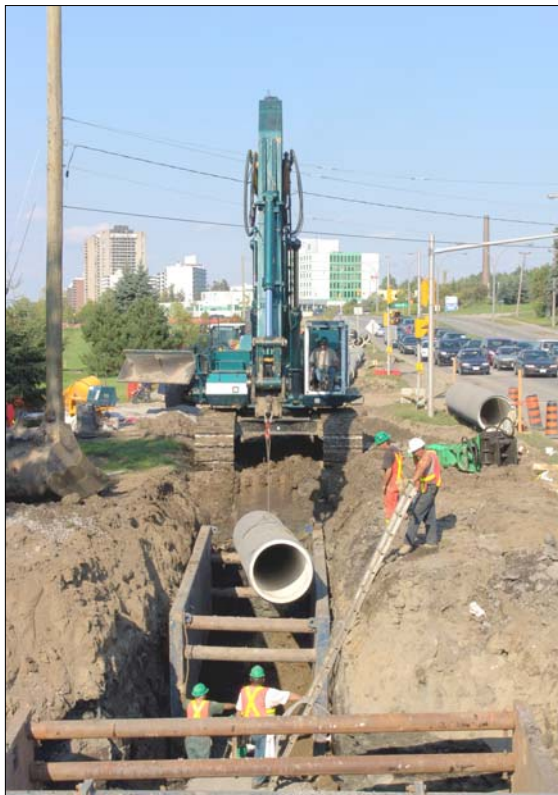
A section of the prestressed concrete cylinder pipe being lowered into the trench.
