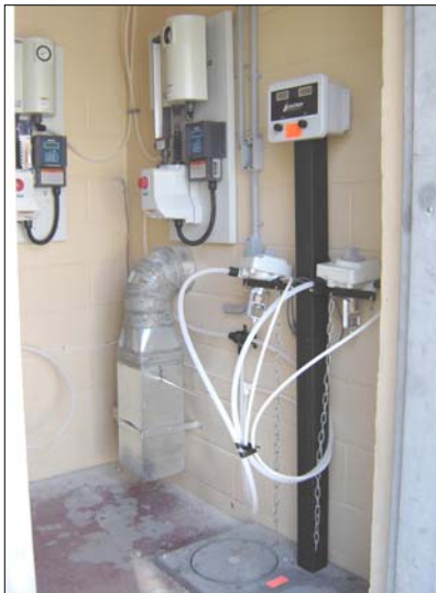
Inside the chlorine room at the Anne Street reservoir showing the chlorinators, weigh scales, vent and gas sensors.
