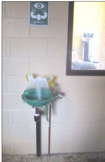
The emergency eye-wash station on the outside wall of the chlorine room.
