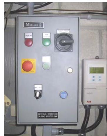
Bayfield Street booster-pump control and monitoring equipment.
