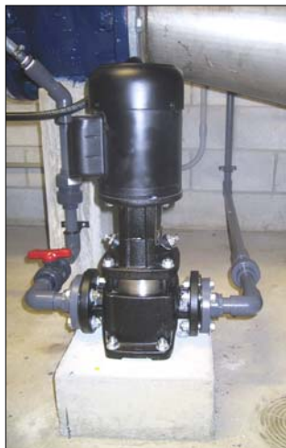
The chlorine booster pump at the Bayfield reservoir showing the water draw and injector piping.
