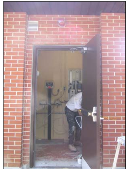
The dedicated access door to the chlorine room. The emergency strobe light and exhaust vent can be seen above the door frame.
