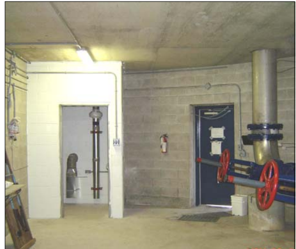
Completed chlorine room inside the valve room at the Mapleview Elevated Tank Reservoir.
